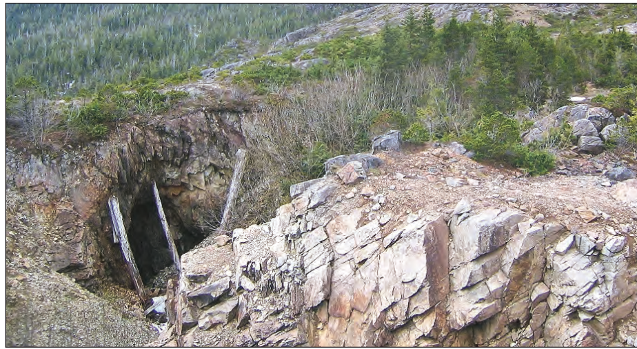
A study completed for the U.S. Forest Service recommends filling the 300-level portal (above) and two other underground mine openings at the historic Ross-Adams uranium mine with concrete.
