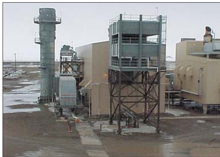
Gas-driven turbine generator, built to meet future Kuparuk River unit needs
