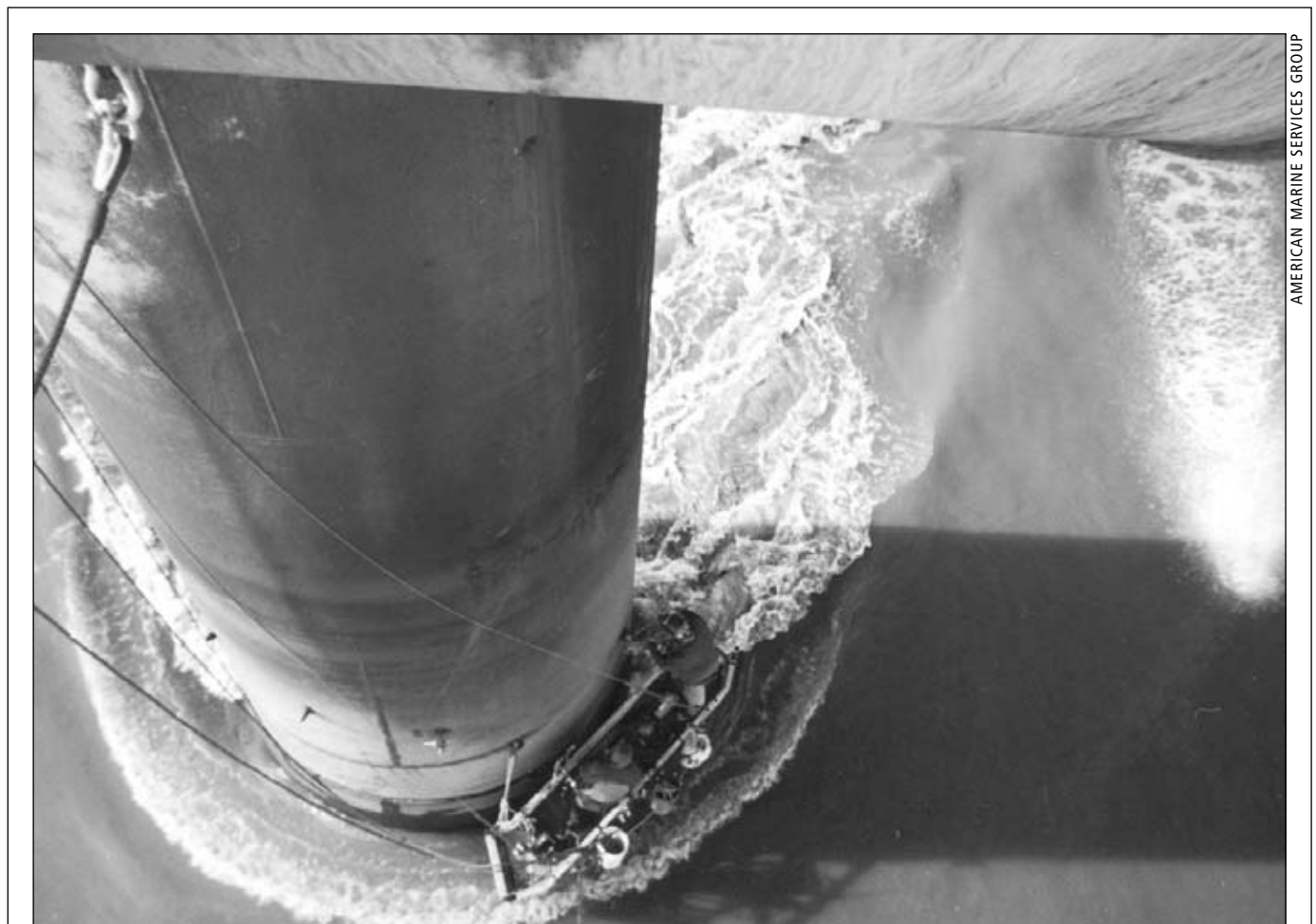
Workers with American Marine Services group perform maintenance duties on a Cook Inlet platform. Along with regular company profiles, this month's Petroleum Directory features additional photos of the companies profiled.
