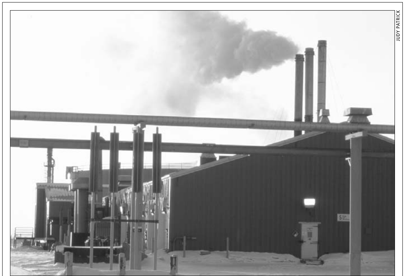
Pump Station 1 at Prudhoe Bay on Alaska's North Slope. The original pump station design was driven by what was needed when the pipeline was built, and by the fact that there were 2 million barrels of oil a day to move, versus the 1 million barrels being moved today. (See stories on Alyeska Pipeline Service Co.'s strategic reconfiguration in the July 6 and July 13 editions of Petroleum News.)
