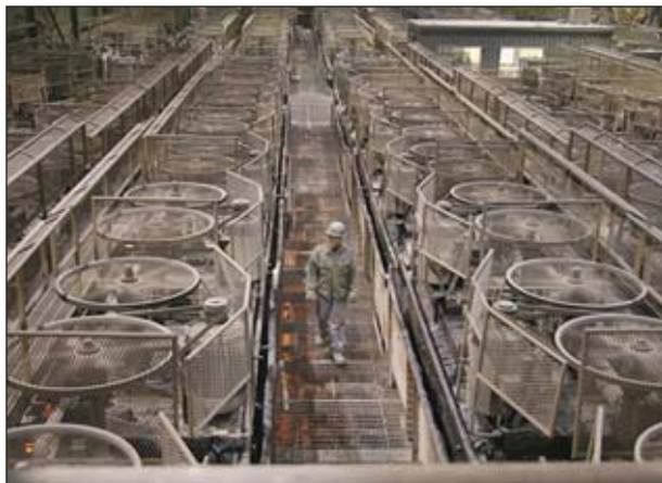
The operators of the Endako Mine in British Columbia aim to improve processing efficiency in the mill and roasting facility by upgrading major processing equipment.
