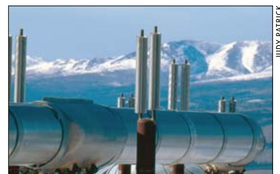
The trans-Alaska oil pipeline
