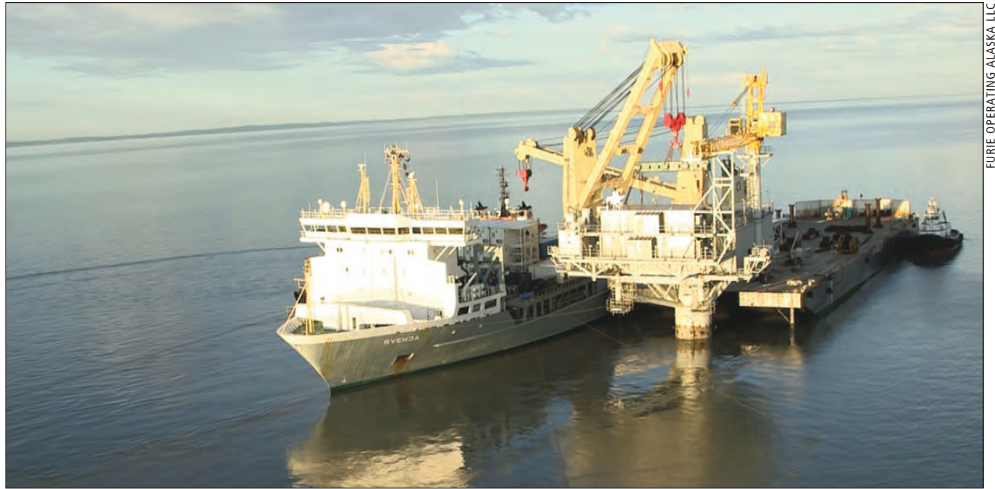
The MV Svenja positions the topside deck on the monopod caisson of Furie Operating Alaska's Kitchen Lights gas production platform.
