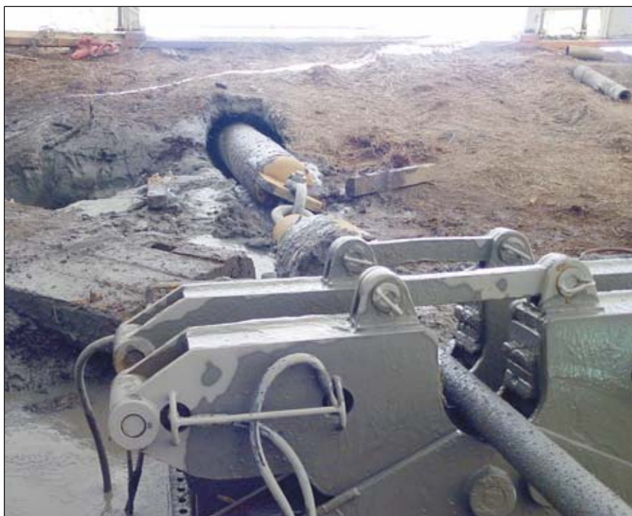
Pipe exiting after being pulled through horizontal directional drilled crossing under channel
