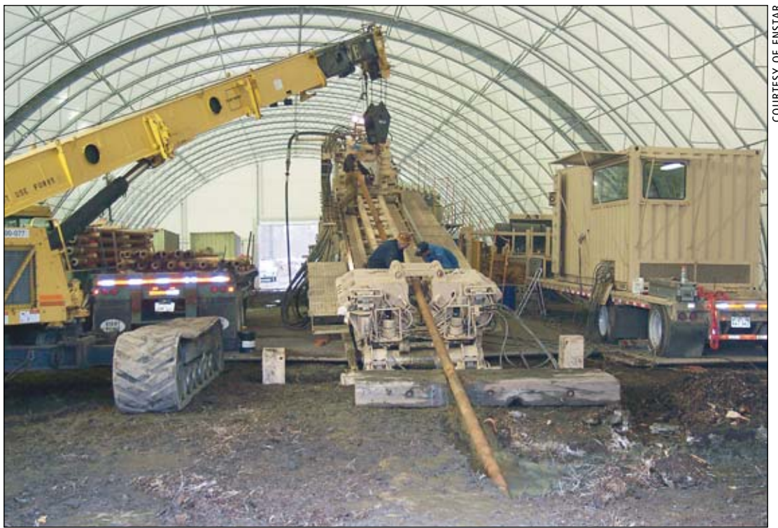
Horizontal directional drilling at the middle channel crossing of the Big Susitna River
