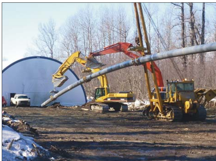
Sections of 20-inch natural gas transmission pipe have been welded together and are being pulled through the drilled and reamed hole
