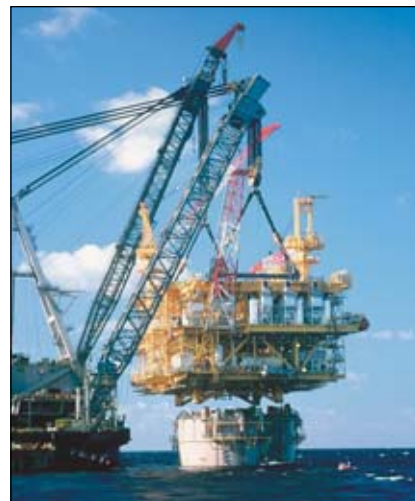
J. Ray McDermott's DB50 and Shear Leg Crane perform the dual lift of the 6,220 short ton topsides on the Front Runner Spar hull.
