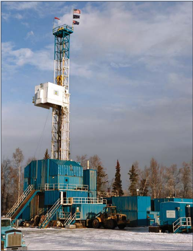
Linc Energy recently completed LEA No. 1, pictured above, its first exploration well in Alaska. The Australian company drilled the 6,323-foot well in the Point MacKenzie area.
