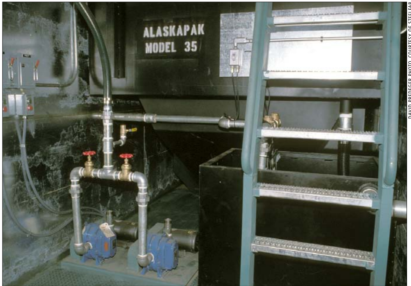
Another view of the ALASKAPAK water and sewage treatment plant fabricated by STEELFAB. Ideal for remote locations, the ALASKAPAK can be fabricated for any size of community. See the company profile on page B13.
