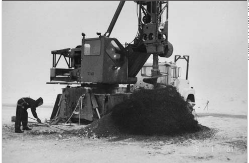
Morrison-Knudsen Co. and NANA Development Corp. did construction for ARCO Alaska Inc. Here a drill rig bores hole for pipe supports on Kuparuk River crossing.
