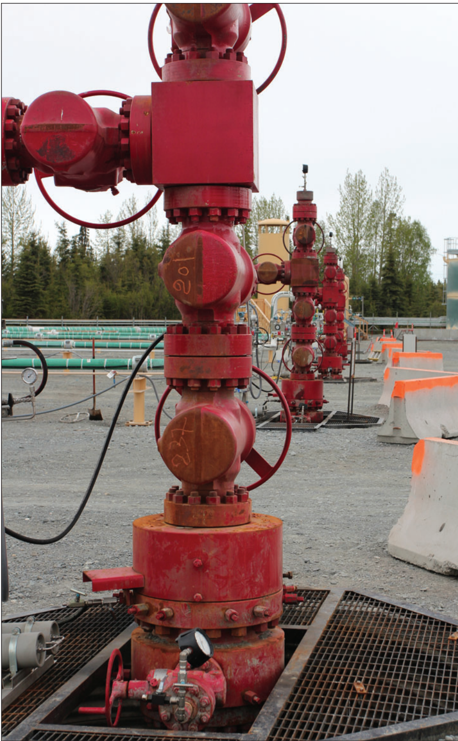
Wellheads in the Cook Inlet Natural Gas Storage Alaska facility on the Kenai Peninsula.
