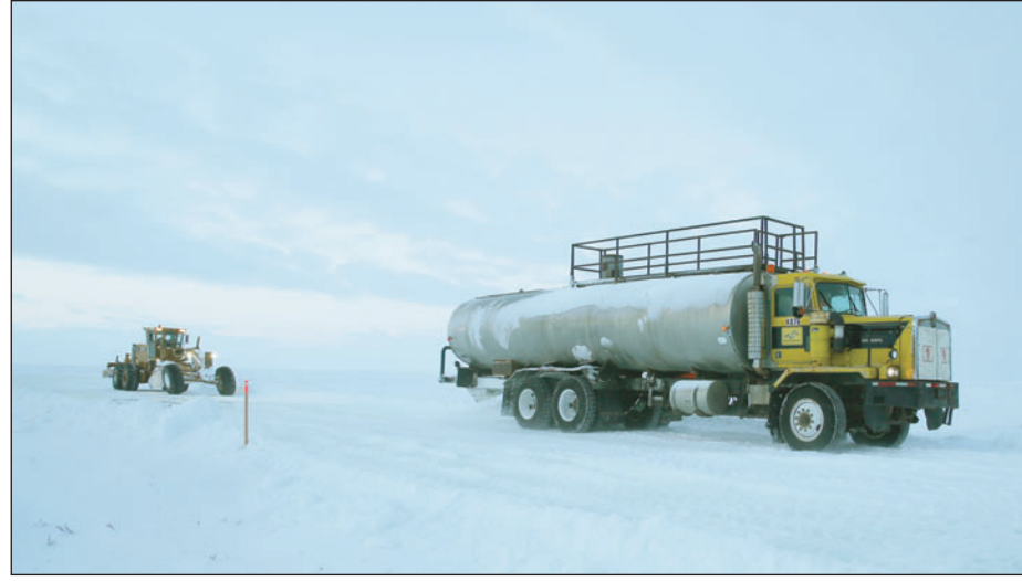
Road access is one of the greatest challenges to development on Alaska's Western North Slope; ice road construction at Willow.
