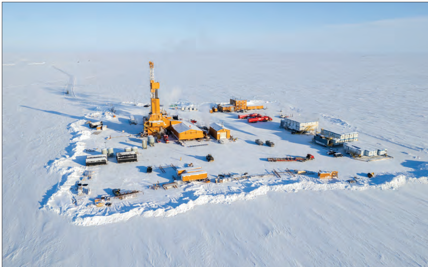
King Street #1 Well Pad and Ice Road, Lagniappe Project, North Slope Alaska, Armstrong Oil & Gas, Inc.
